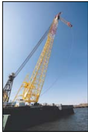
The Chesapeake, a 1,000-ton lift capacity derrick barge, the Ferrell, a 200-ton lift capacity revolving crane barge, and the Oyster Bay, a 150-ton lift capacity crane barge are being used by the Navy's Supervisor of Salvage and Diving to remove submerged portions of the Francis Scott Key Bridge. U.S. Navy photo by MC2 Hannah Mohr
